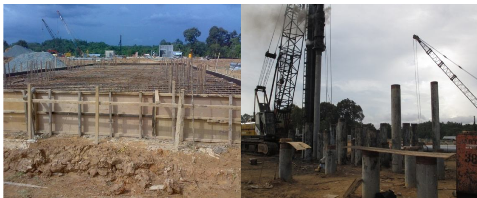
Fig. 4. (a) Side view of stack, (b) pile cap reinforcement, (c) pile layout, (d) piling in site, (e) pile cap was ready to concreting
