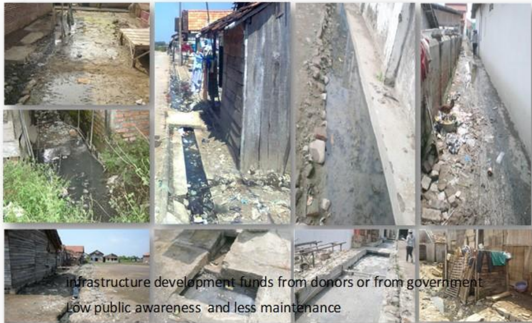
Figure 6 Drainage Condition Source: Observation and in Depth Interview, 2015
