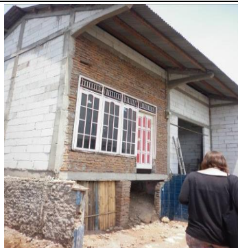
Figure 13. One of the houses to be elevated due to a decrease in soil
