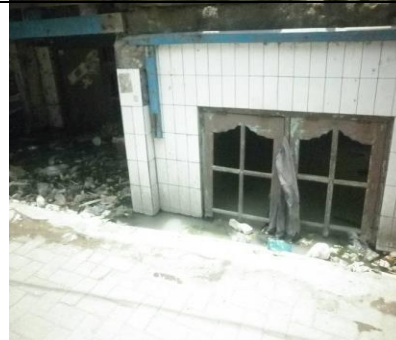
Figure 14. The house should be abandoned because it was submerged by water
