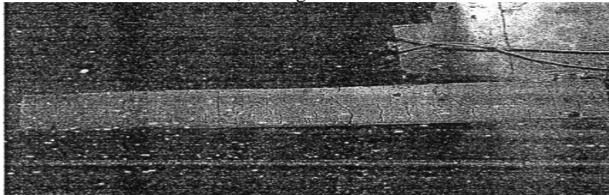
Figure 10. The crack pattern and collapse type of Reinforced Concrete Beam with 2 Tensile Reinforcements
