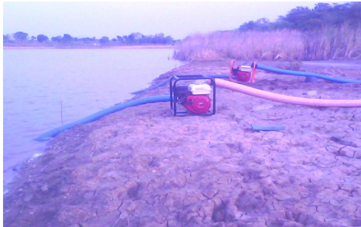
Fig. 2. Swamp Water Intake in Setro
